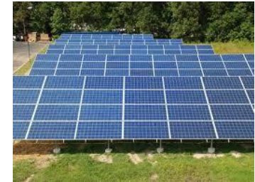
Panels Making Up An Array
