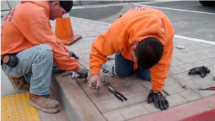
24. The treads of the L-Bolts are cleaned in preparation for mounting the pole base.
