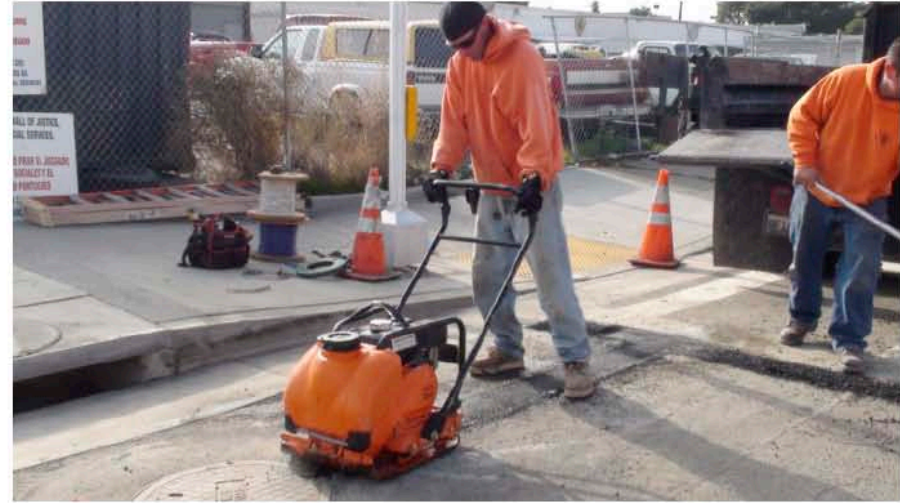
39. An asphalt compactor is used to finish the leveling and smoothing of the asphalt.
