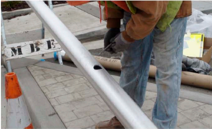
26. Access holes are cut into the pole at various locations to provide access for Electrical cabling between system components.
