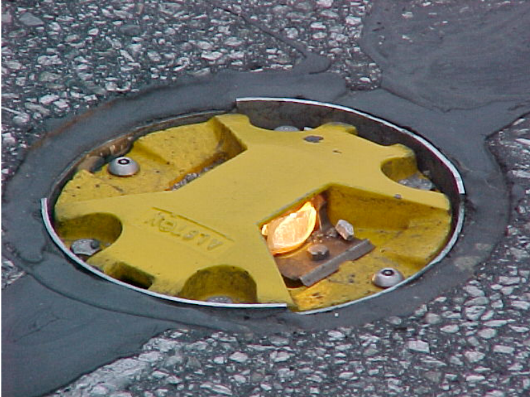
FIGURE 4 Installed in-pavement flashing warning light.
