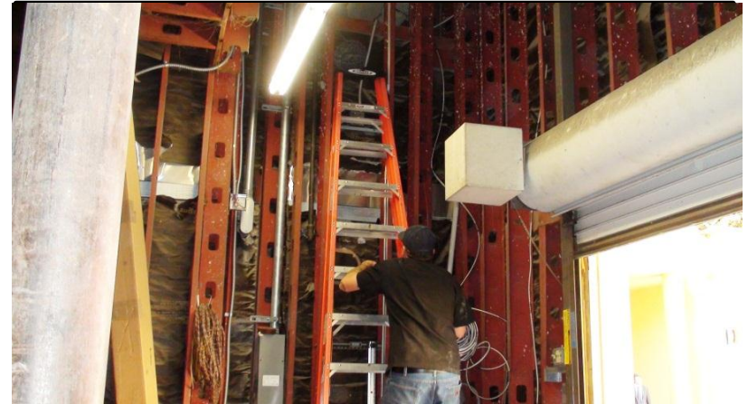
Figure 30: Wiring from the Second Sign being Routed Down to the Controller Enclosure Location
