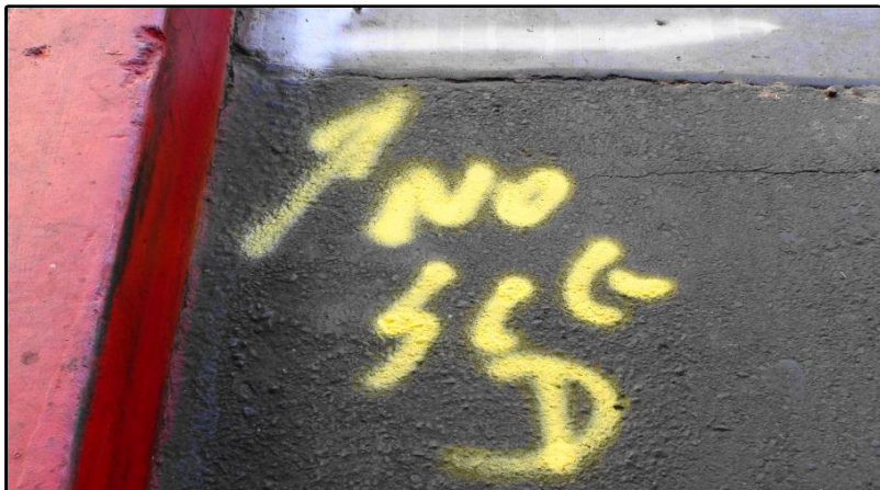
Figure 11: APWA Color Code, Yellow = Gas Line, Companies Such as “DIG ALERT” and “Underground Service Alert” can Locate all Utility Lines
