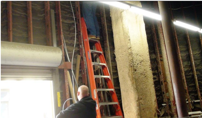
Figure 27: Wiring from the Sign is Routed through the Overhead Archway and Supporting Columns
