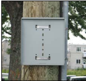
Figure 9: Pole Bracket banded to utility pole
