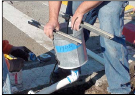
Base Can Attached to Drain Conduit
